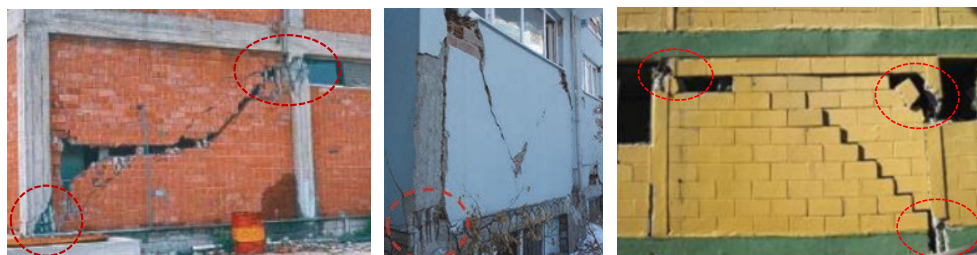
Figure 3. Cracks and crushing of infill and columns in an earthquake as a consequence of mutual action: a) Adana-Ceyhan earthquake 1998 [1]; b) Van earthquake 2011 [1]; c) Chile earthquake 2010 [12].
