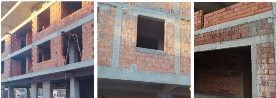
Figure 1. RC frame structures with masonry infill: a) unanchored walls; b) walls anchored with vertical cerclages; c) walls anchored with horizontal and vertical cerclages. Case studies from Banja Luka, Bosnia and Herzegovina. Photography by authors, 2024.
